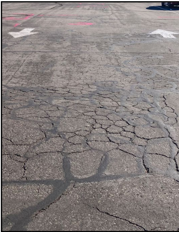
IMAGE 1: Alligator cracking at entrance to east side of parking lot
