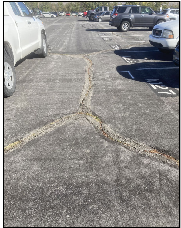
IMAGE 2: Previously sealed cracking at TH-3
